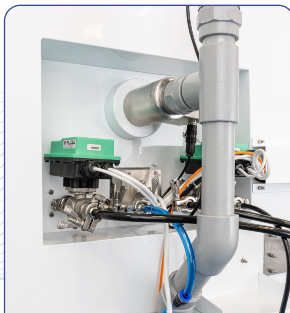
Close up of VHP injection pipework at rear
