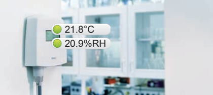
Live data showing the conditions overlaid on actual environment photo
