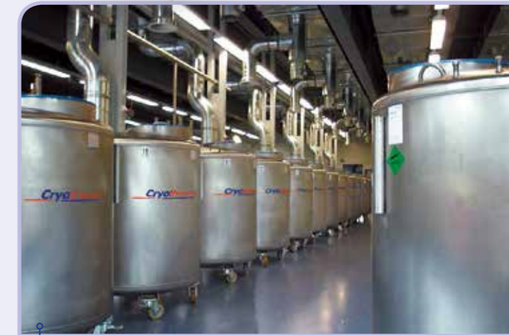
Cryogenic facilities with > 100 freezers © Photo Fraunhofer IBMT, Dr. Obergrießer
